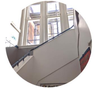
Damp damage to existing wall to stairwell
