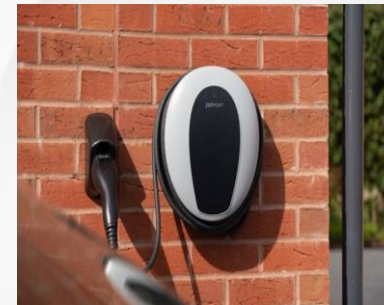
EV Charging Points
